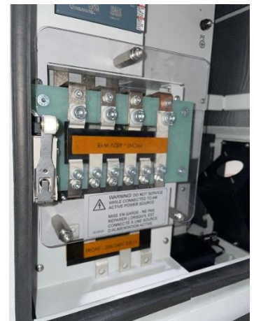
Figure 18 — Spare configuration bus bars, Delta and Single, anchored together in storage area
