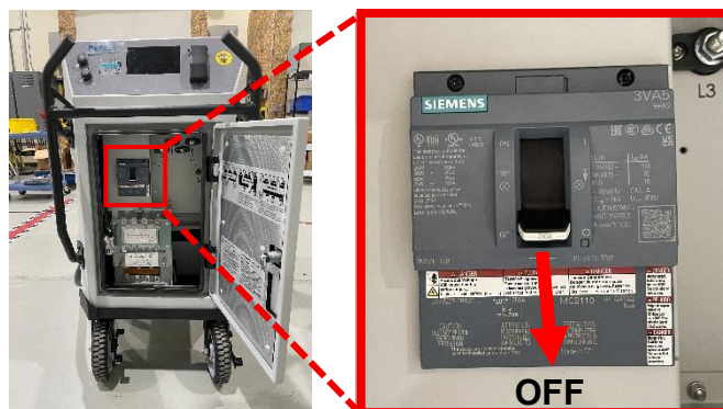
Figure 5—AC main power switch in the OFF position
