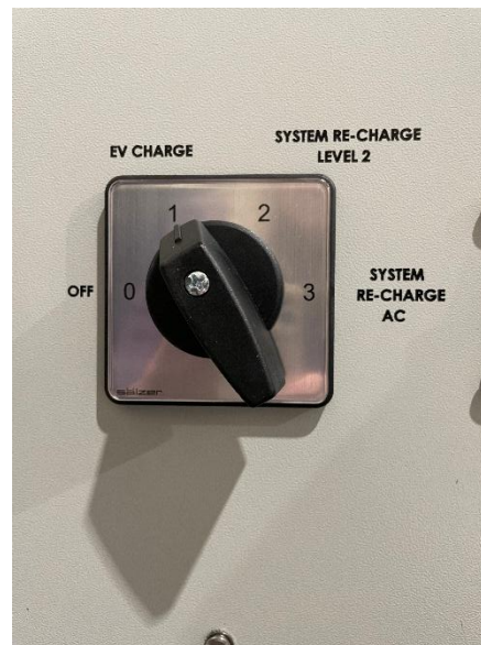
Figure 9—Selector Switch in EV CHARGE (1) position
